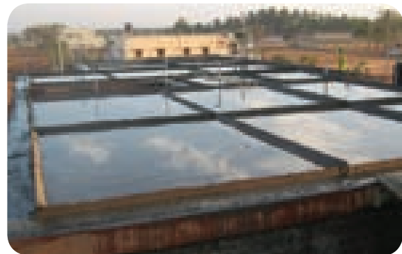
Ponding with water
