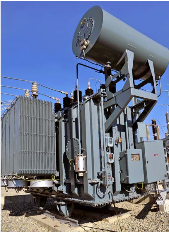
Fig 6.13 Protective devices of transformer
