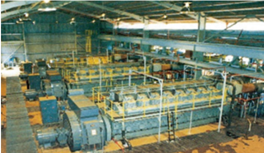
Diesel Power Plant
