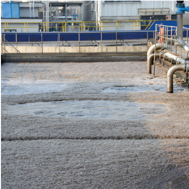
Sludge treatment and disposal
