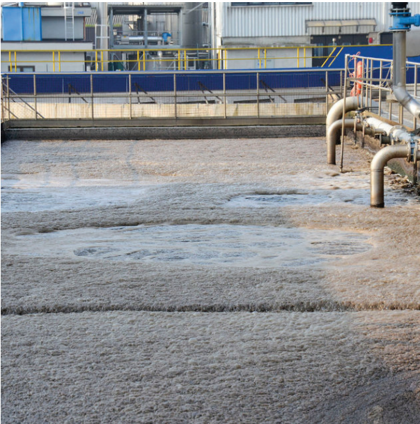
Sludge treatment and disposal
