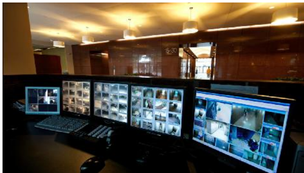
Plate 1.8 CCTV Security System Monitor with Multiple Camera Views of Hotel
